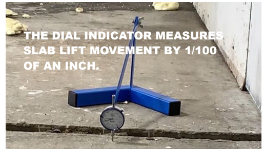
INJECTION OF AP LIFT 430 BEGINS AT THE POINT ABOVE THE LARGEST VOID
